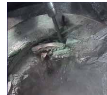
The upper ring of the crucible is to remove with a air hammer.
