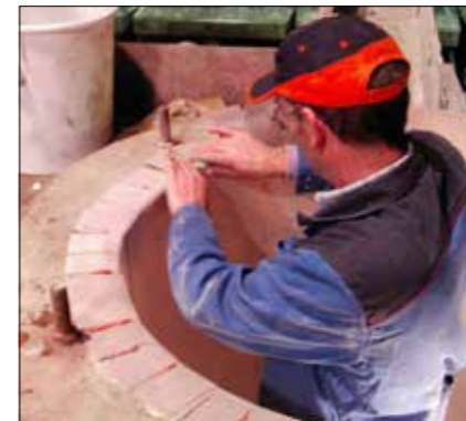
Before inserting the DORIT prefabricated crucible, first install the insulation and the floor-molded bed for the crucible.
