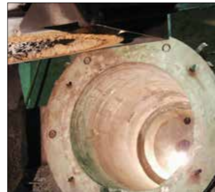
The furnace is to clean and the coil grout is to check
