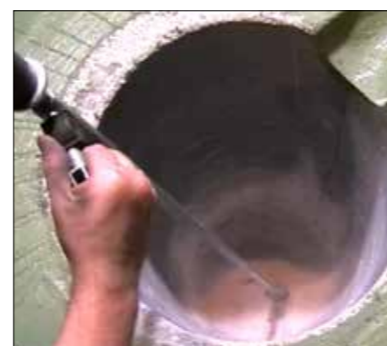
The assembly opening is to fill with special hole mix and to vibrate.
